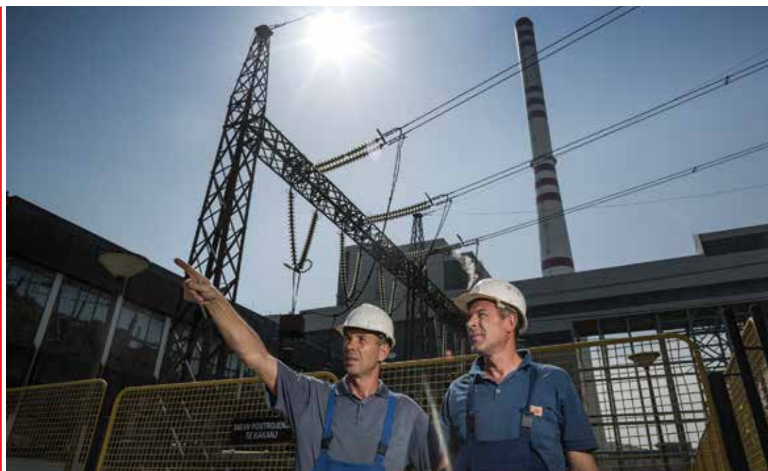
Thermal Power Plant Kakanj
