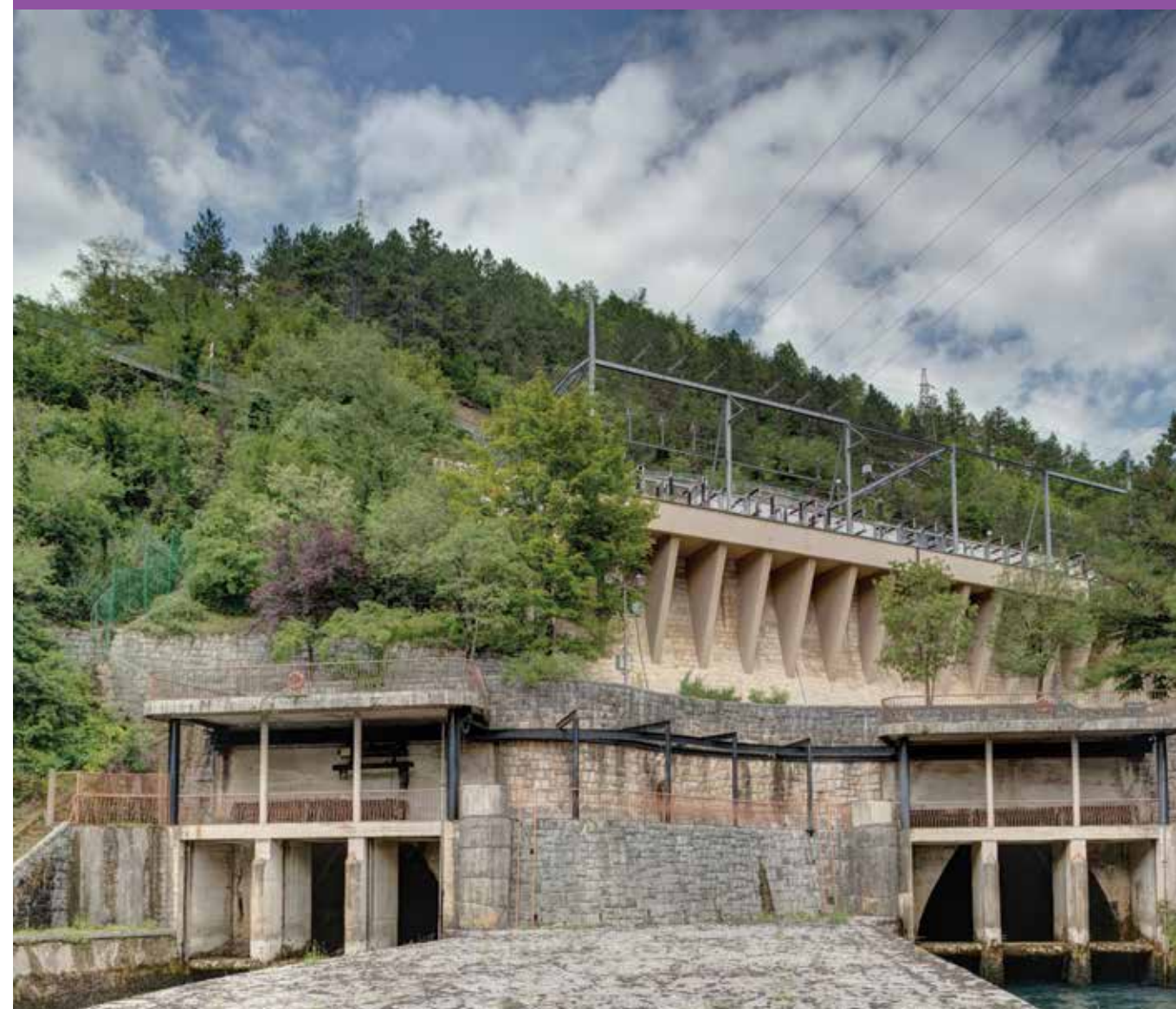
Switchyard of Hydro Power Plant Jablanica
